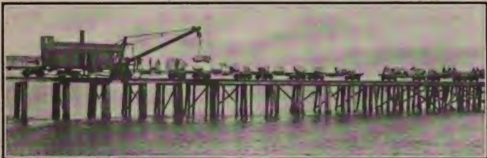
The rocks of granite which are being lowered to form the superstructure, weigh from eight to twenty tons
